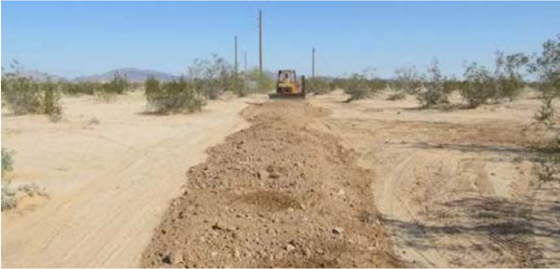
The Road to Ogilby Campground.
